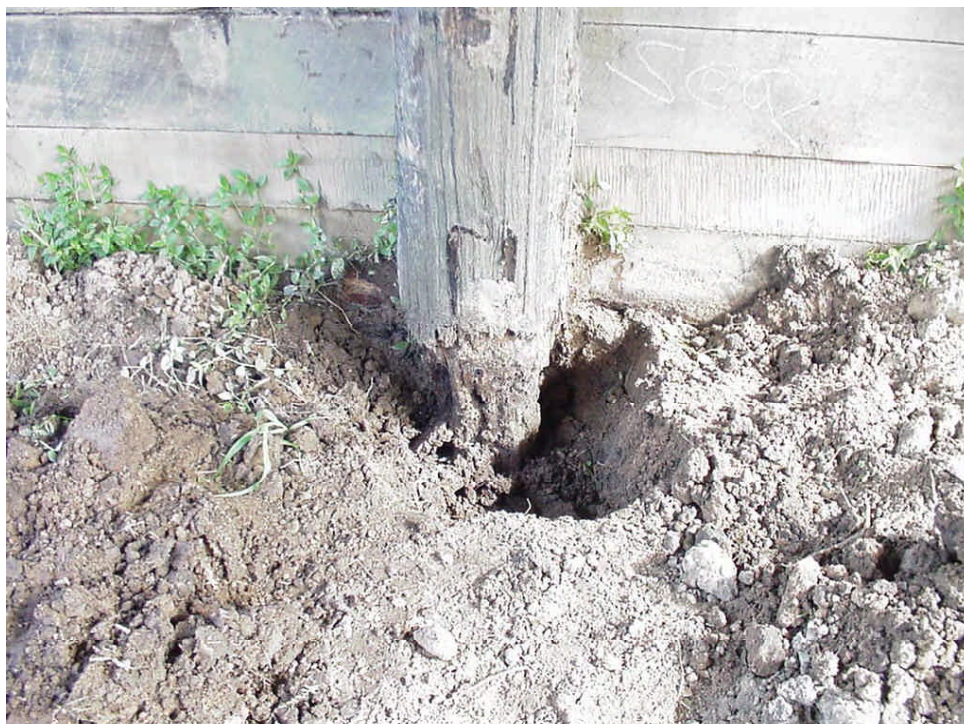
Significant rot and major loss of section just below the ground surface.
