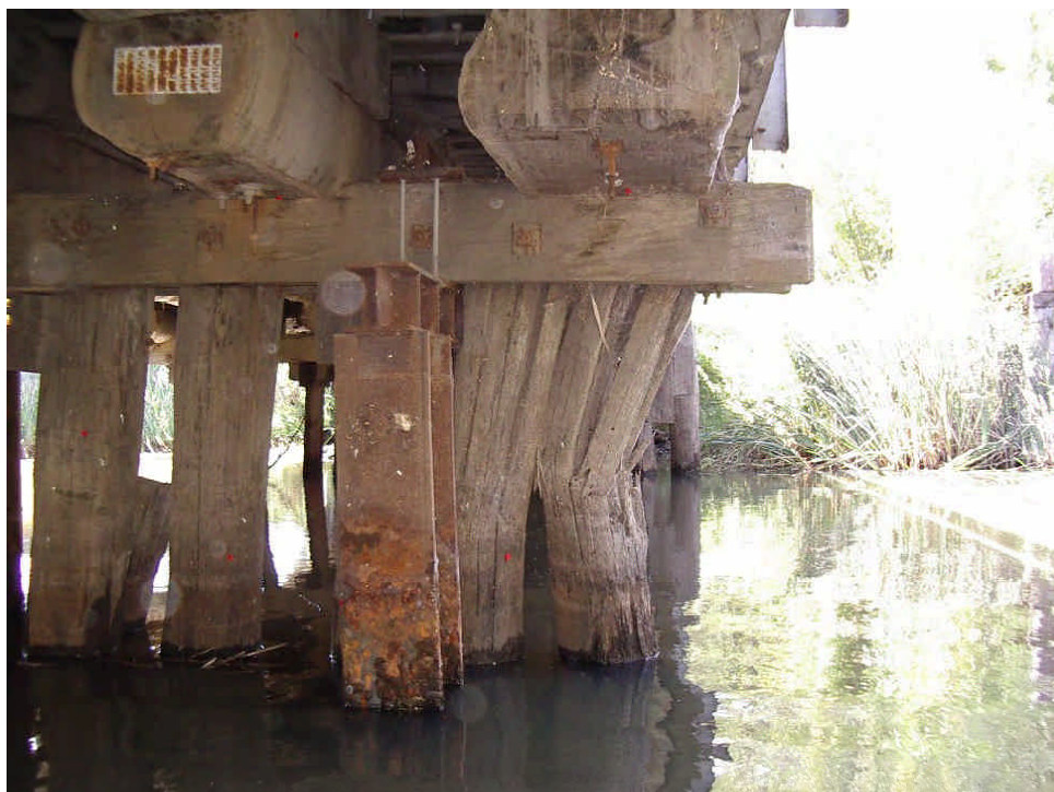
Failed timber piles.
