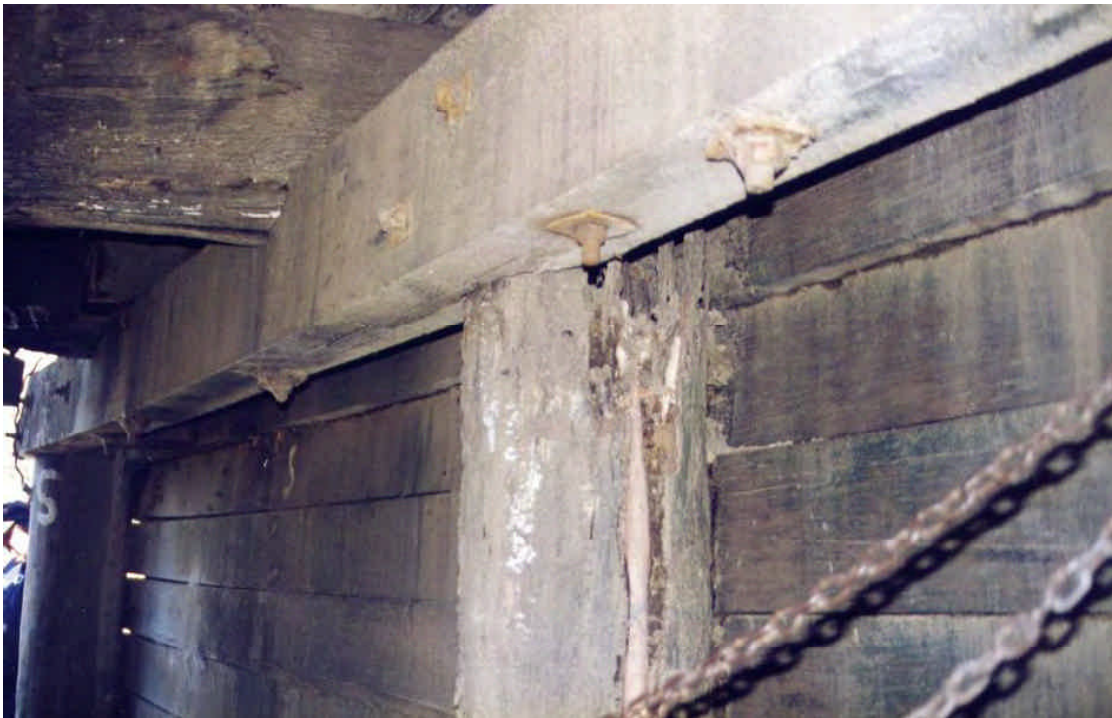
Badly rotten pile.
