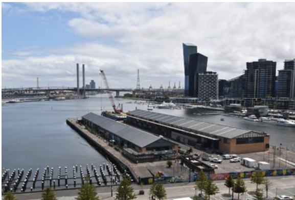
Figure 25. November 2023 view of Central Pier showing the commencement of demolition. Source: Development Victoria, November 2023.
