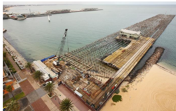
Figure 24. View of the 'sea of piles' at Princes Pier where the deck of the pier was not reconstructed following conservation works. Source: Major Projects Victoria (Peter Glenane).
