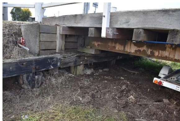
Figure 17. Detail view of new steel girders under Kirwans Bridge. Source: Extent Heritage, 2022.
