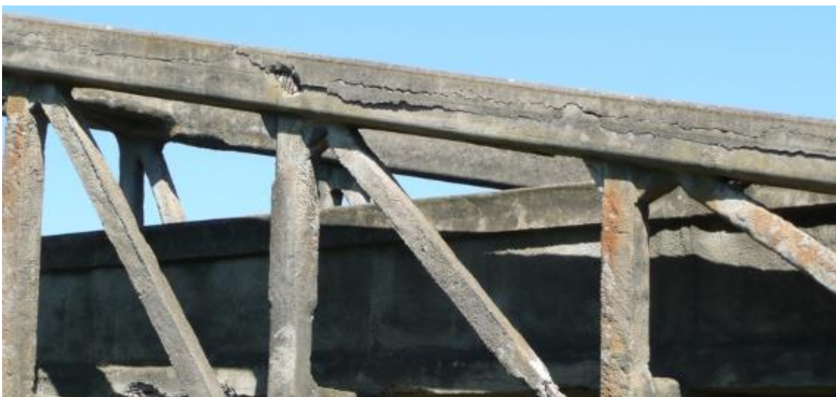
Figure 22. Detail of the bridge showing concrete deterioration. Source: Heritage Victoria, 2020.
